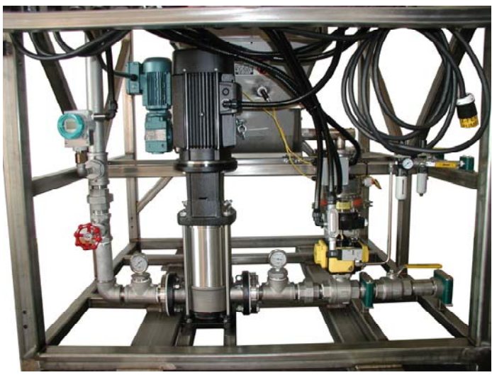
Dilution Water Handling System
