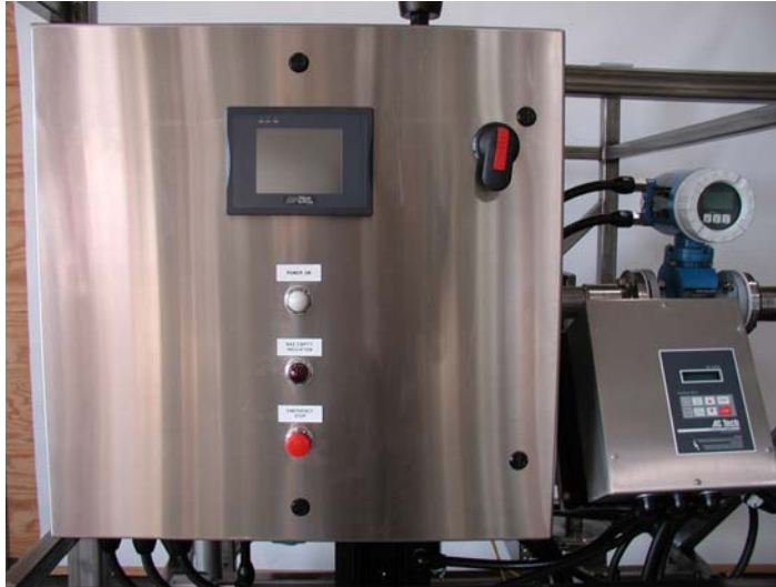
EGM Designed PLC Control Panel
