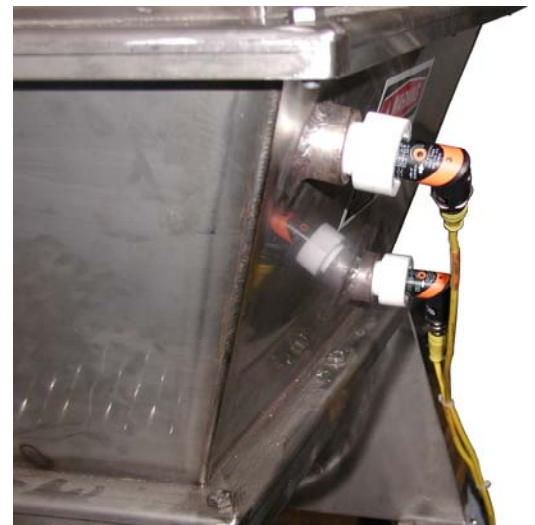
EGM Dry Chemical Feed Unit Hoppers
